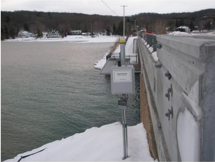
Photo 2. The solar panel, data logger, and modem at the narrows. The pressure transducer (calibrated to read water height above sea level) is in the channel about 3 1/2 feet under the surface.
